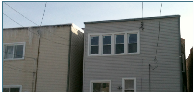
Liz Vogel's home (above, right) is now free of the ice dams seen on a neighboring building (above left).
