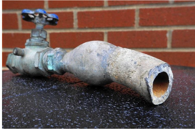
The cost to replace a LSL varies by community and on the length of the pipe from the building to the water main. Photo from Associated Press.
